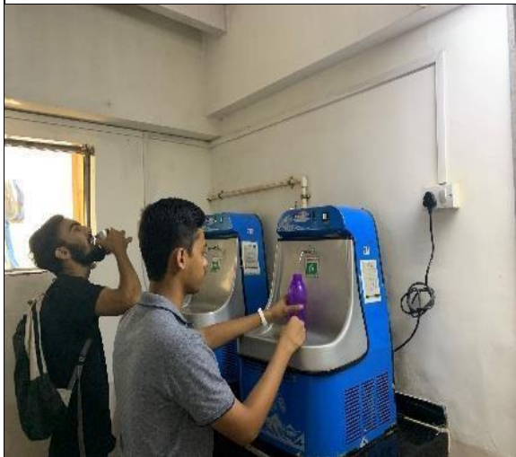
Drinking water facility
